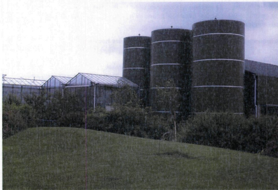
Heat storage tank" or (heat) buffer
