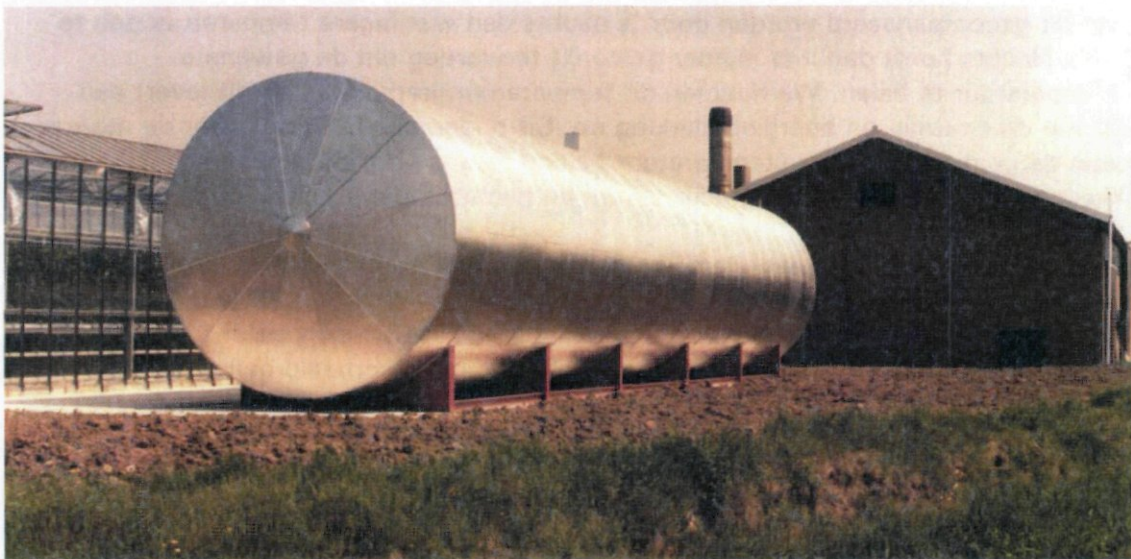
Heat storage tank or heat buffer
