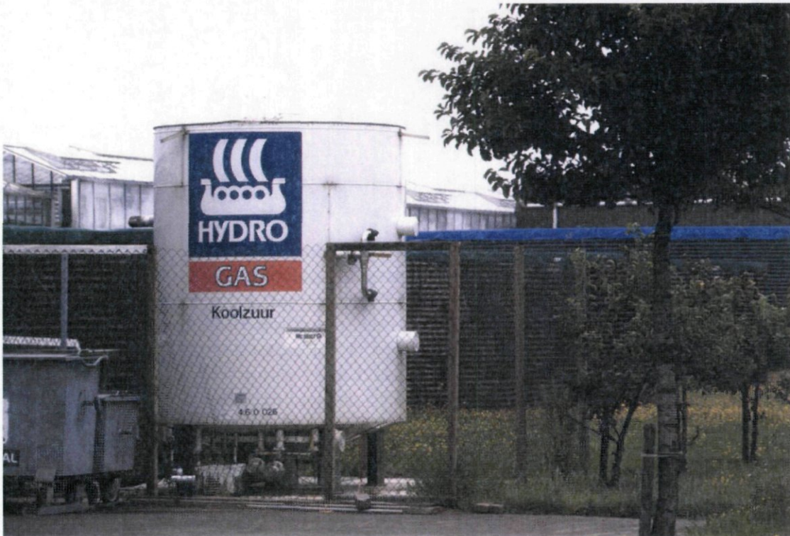
Storage tank for pure CO 2 (cryogenic tank)
