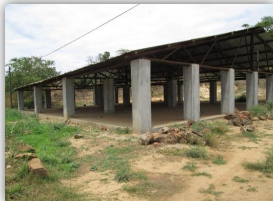
Picture: Construction of a new market building on the Nobeza Nolta market, Manica.
