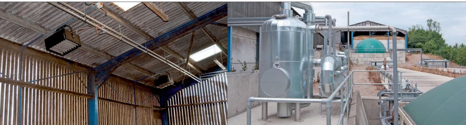
Central heating: water generated by AD is used to heat calf housing Power plant: Broom House Farm's anaerobic digester
