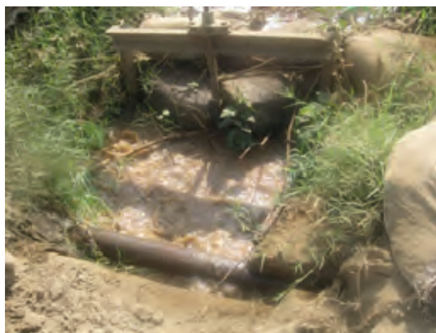
Figure D.6. Gemoia offtake structure at low irrigation demand closes by sacks
