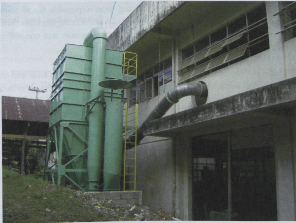
Figure 44 The air cleaning system
