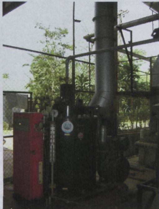
Figure 42 The steam generator
