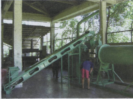
Figure 36 The covered transportation belt
