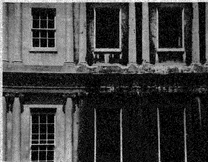
Fig. 4. Blackened and corroded stonework in the English city of Bath in Somerset, the result of domestic pollution. The building on the left had recently undergone costly restoration.
