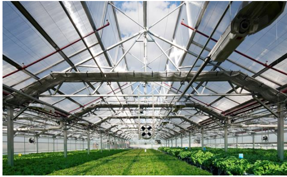
Figure 4 CEA production system
