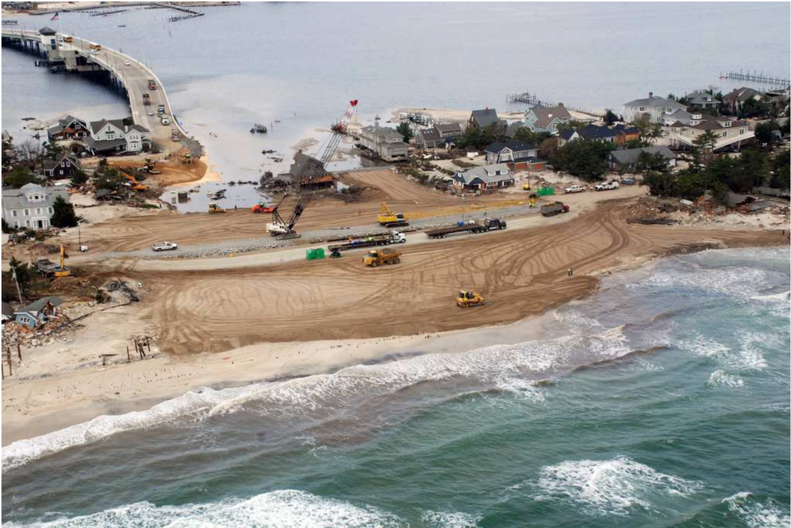
Photo courtesy of U.S. Army Corps of Engineers Superstorm Sandy levee repair in Montoloking, New Jersey :
