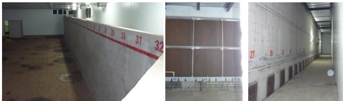
Figure 5.5. Pictures inside of McCain storage facility (April 2014).
