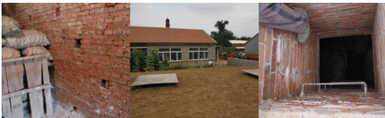
Figure 5.2. Horizontal ventilation ducts in a tunnel store (left), top view of a pit store (middle) and top an opening of pit store for loading and unloading (right).
