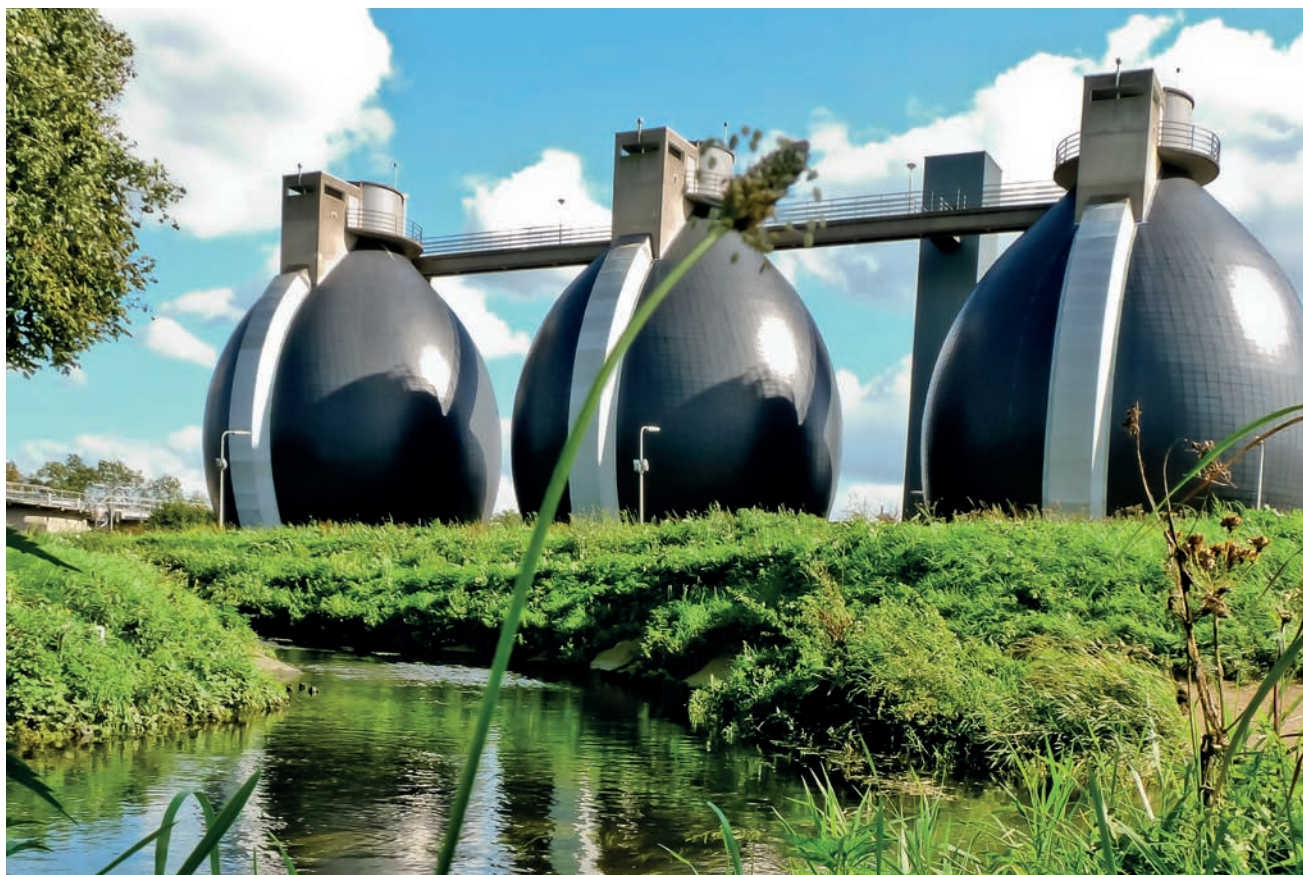
Figuur 1: Vergistingstanks rioolwaterzuivering
