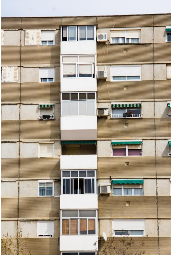
Image 21: Deterioration of buildings (2)
