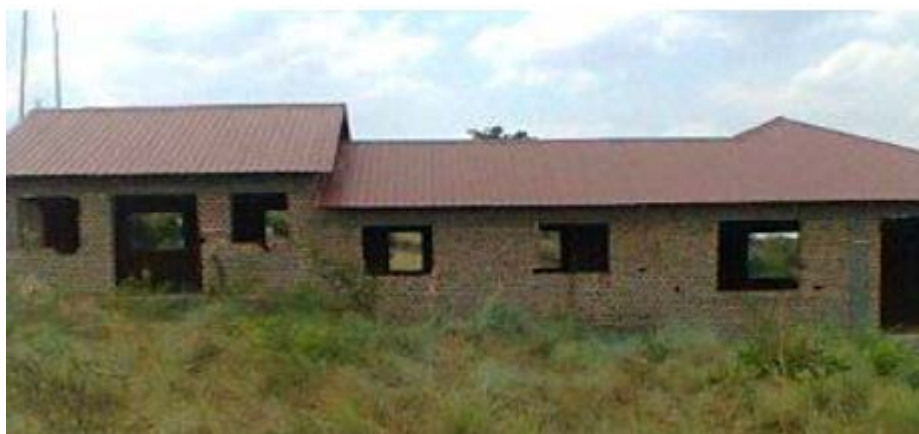
The cooperative building under construction. The building has proposed Board room, cooler room, Agro-vet- store and offices.
