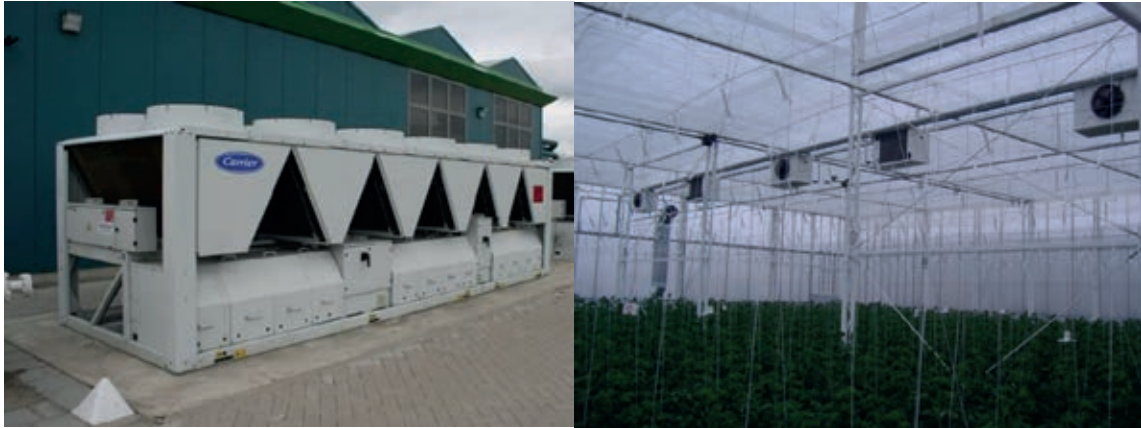
Figure 5. Cooling installation outside and inside the greenhouse needed to remove the heat in a closed greenhouse. This type of greenhouse is considered high-tech.
