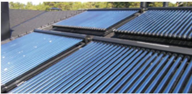
4.8 Solar collectors (Saulessiluma)
