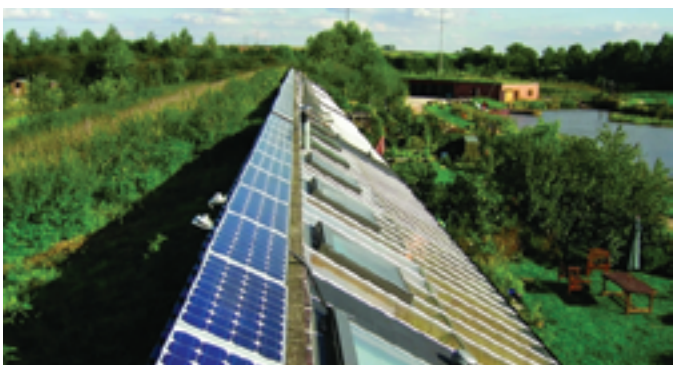
7.36 Very sustainable housing with solar panels on the roofs (Soullife)
