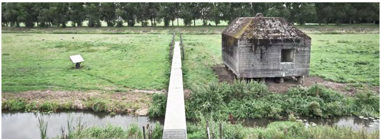
Figure 2.12. Foundations of an old defense bunker revealing the ongoing soil subsidence in the Vechtplassen
