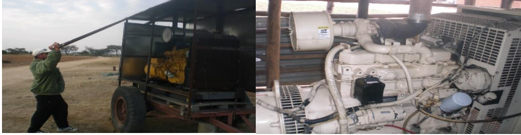
Figure 5.3. A producer showing two generators available at the farm with one standby generator to the left. Source: (Author, 2013)
