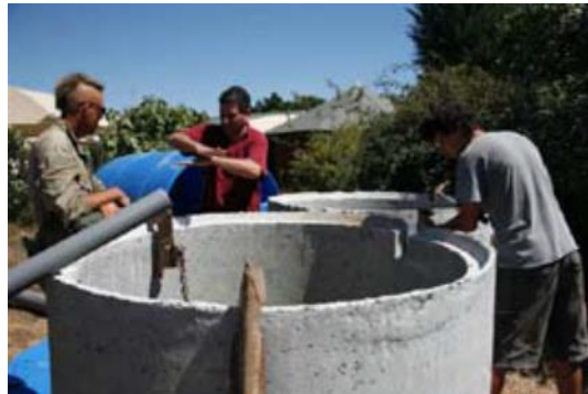
Figure 6.5. A simple biogas digester construction at Tamera experimental site (Southern Portugal). Source: (Culhane, n.d.).
