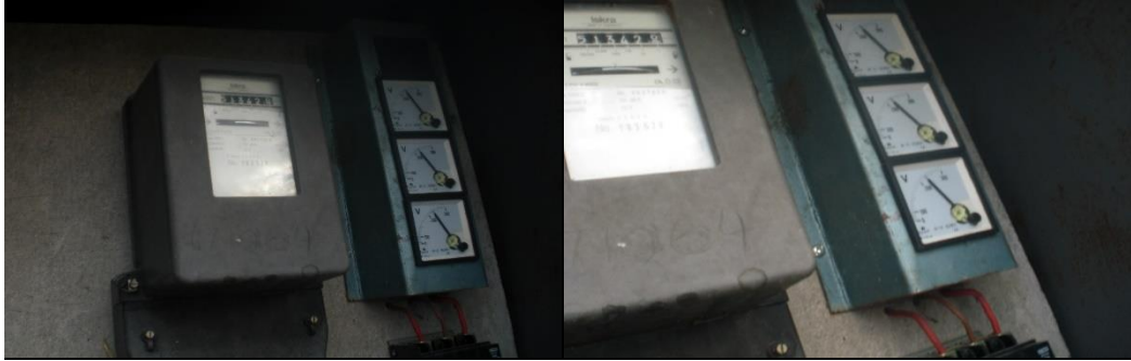
Figure 5.1. Equipment to monitor voltage from the grid. Source: (Author, 2013)
