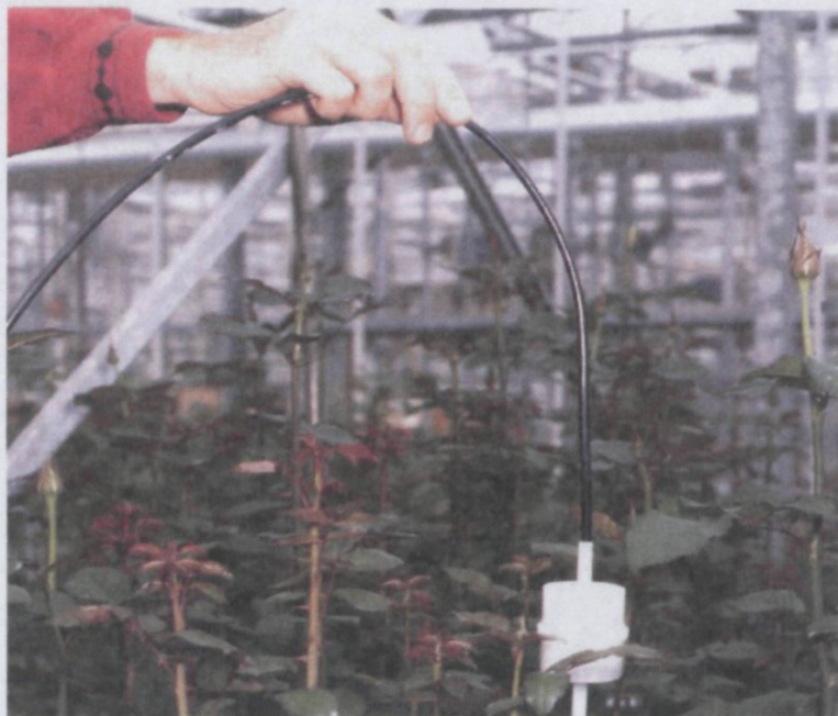
CO 2 measuring point in the greenhouse
