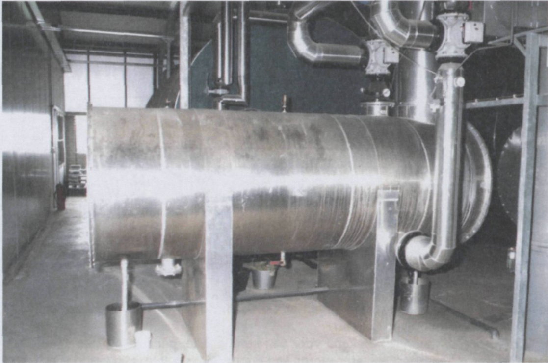
Flue gas condenser
