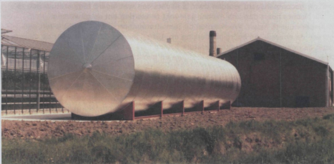
Heat storage tank or heat buffer
