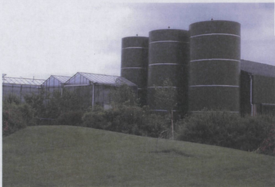
Heat storage tank" or (heat) buffer
