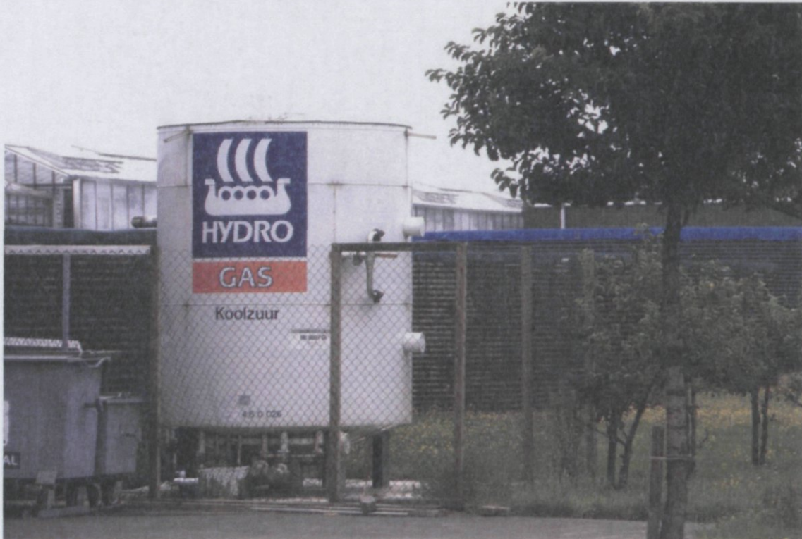
Storage tank for pure CO 2 (cryogenic tank)
