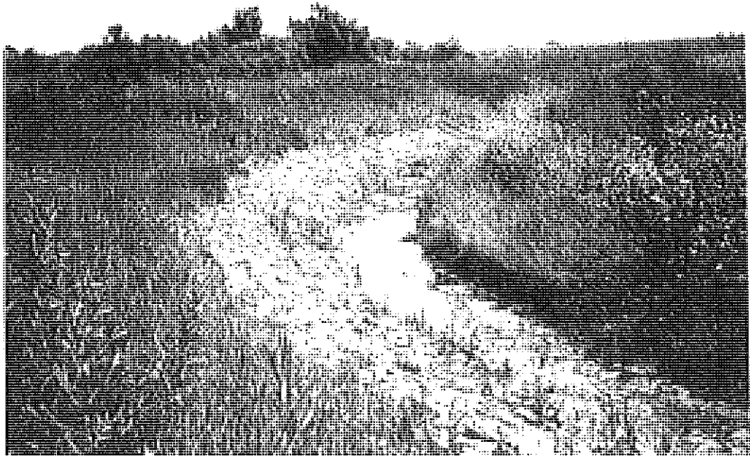
Photo 19.4 The outer curve of a drainage canal may require lining (courtesy, USDA SCS)
