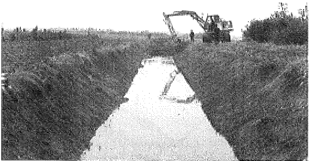
Photo 19.3 This machine can clean a drain with this top-width by working from one side only.
