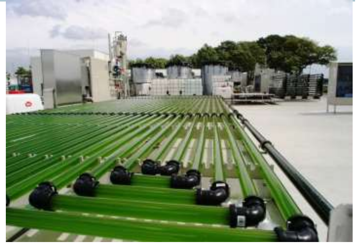
Horizontal tubular reactor
