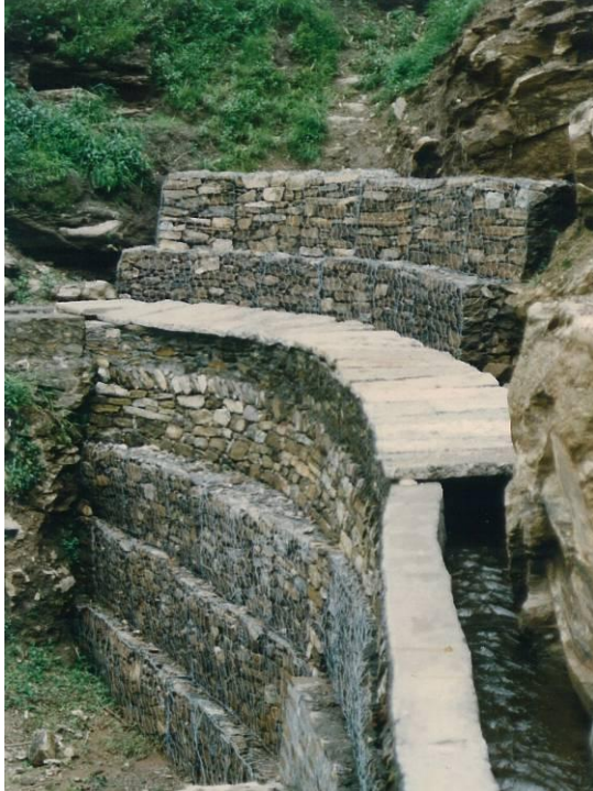
Photo 2: Crossing land slide (1990)
