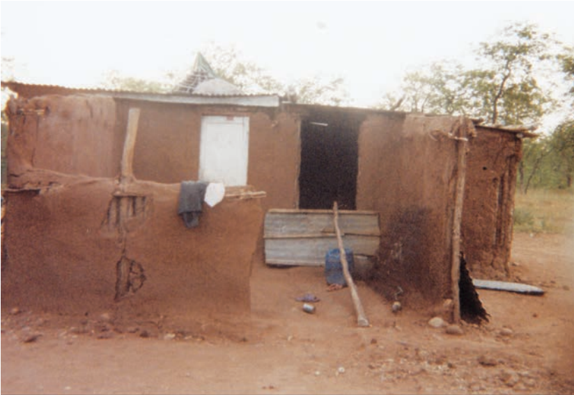
Figure 9.4. Arleta's house in need of repair. 'Since the park was made we were supposed to leave. Since they said that, people don't construct houses, we don't plant trees. This house was built in 2000 but it was never really finished because the park came. There were papaya trees but we stopped planting and the old ones died. No one is investing, so as not to do things for nothing. Even now that we have accepted to leave, the park does nothing.' 83 (Photo credit: Arleta, March 2008)
