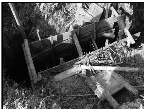
A poorly constructed sluice gate
