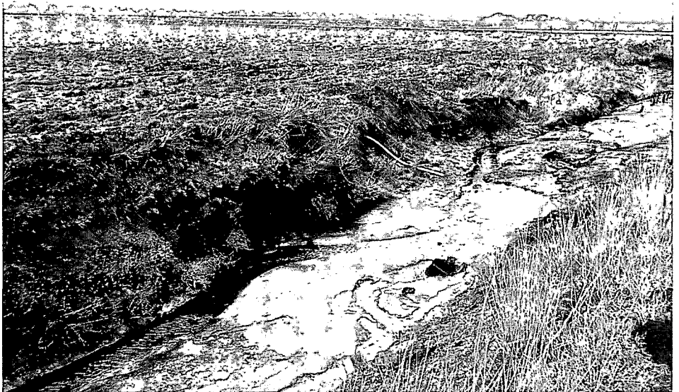
Photo 19.2 Localized failure of a side slope upon construction (Courtesy, L. Molenaar)
