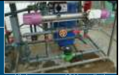
High pressure UV installation
