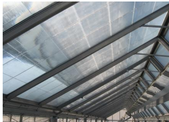
Figure 2: Details of the modular constructed Fresnellens. Each lens is assembled from 12 parts and two lenses are mounted in one double glass pane.
