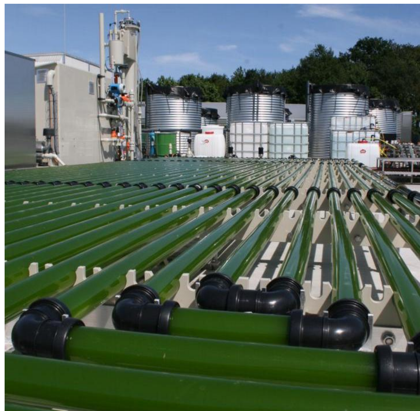
Horizontal tubular reactor
