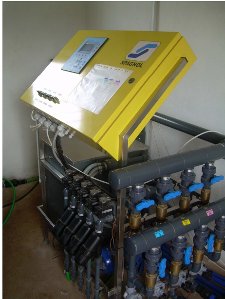
Figure 4 – A fertigation unit installed at the Turkish site (Spagnol Automation, Italy).
