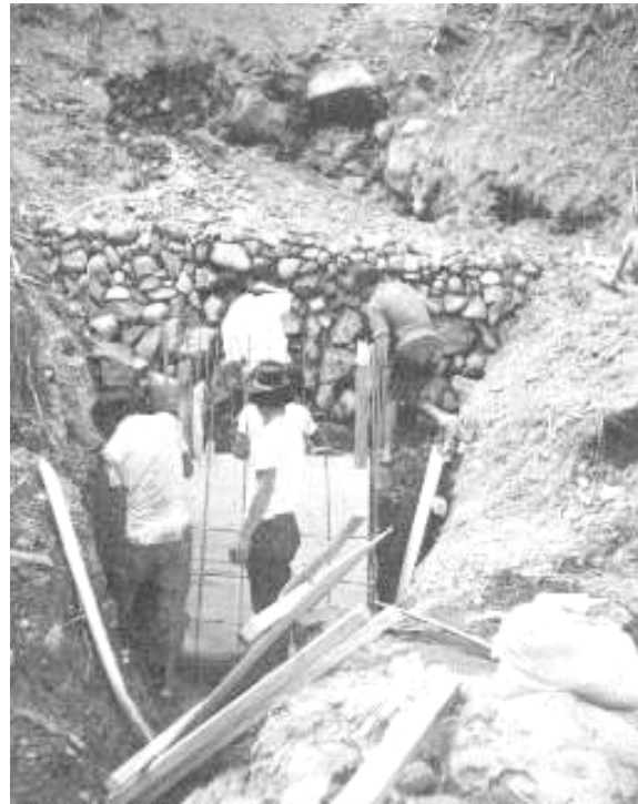
Fig. 1.1 Frantic efforts to prop up the physical structure of the terraces.
