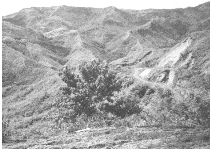
Fig.7.17 Road construction-induced landslides.
