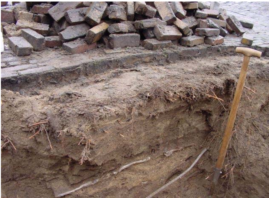
Figure 21 Digging out bags with substrates installed in root zone of no.43 tree
