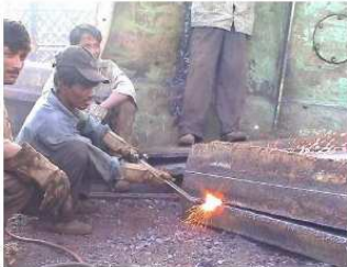
Figure 1. Lacking personal protection equipment
