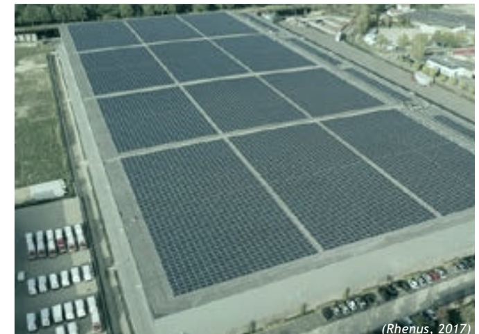
fig 2.42: Solar panels on a distribution centre
