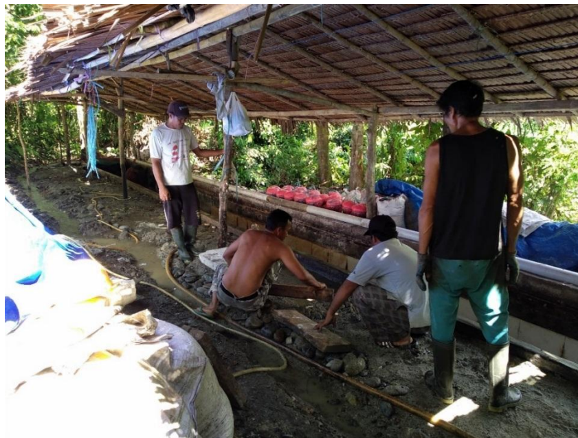
Figure 11. Constructing a permanent floor for the processing place together with in Baliase
