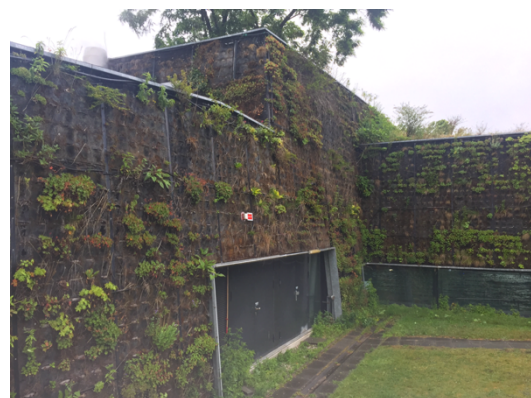
Figure 25 | Failing vertical garden Amsterdam (photo by author, summer 2018)
