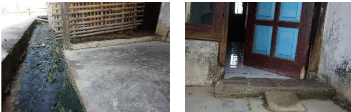
Figure 8 The damage and a precaution action due to flooding hazard (a) After the flood due to different height level between road and settlement, (b) mini water barrier as a precaution
