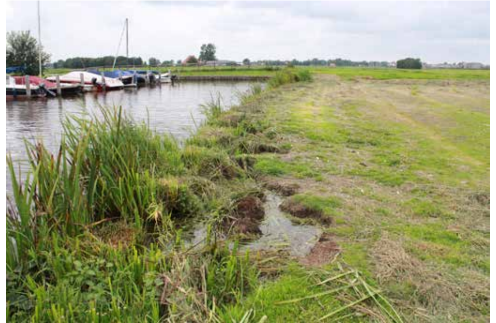
Figure 170 Photo of a damaged local embankment
