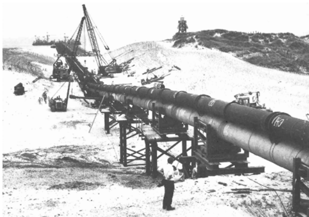
Figure 30: Construction of a pipeline to offshore gas extraction facilities, near Callantsoog. From Borghuis (1988)
