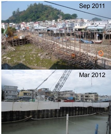
Flood wall in Tai O town – Prepare for the climate extremes on SLR
