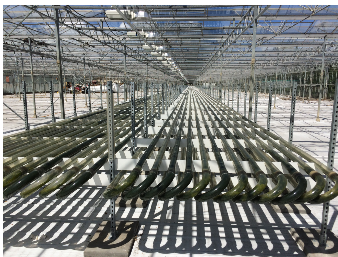
Figure 2-5: Horizontal PBR at LGem (Netherlands)
