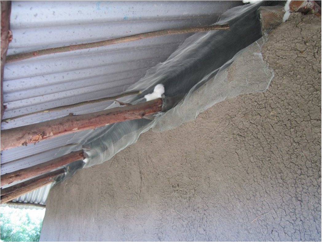
Supplementary Figure 1. Eave screening with wire mesh, experiment I. Wire mesh was applied from the outside. It was first fixed to the lower part of the eave and then stretched upwards towards the corrugated iron sheet roof and clamped around the wooden beams supporting the roof. Gaps between the wooden beams and the wire mesh were filled with cotton wool. To help stretch the wire mesh and hold it flush against the roof, wooden sticks were placed into the eave at regular intervals.
