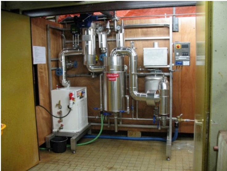
Thermal hydrolysis of waste activated sludge
