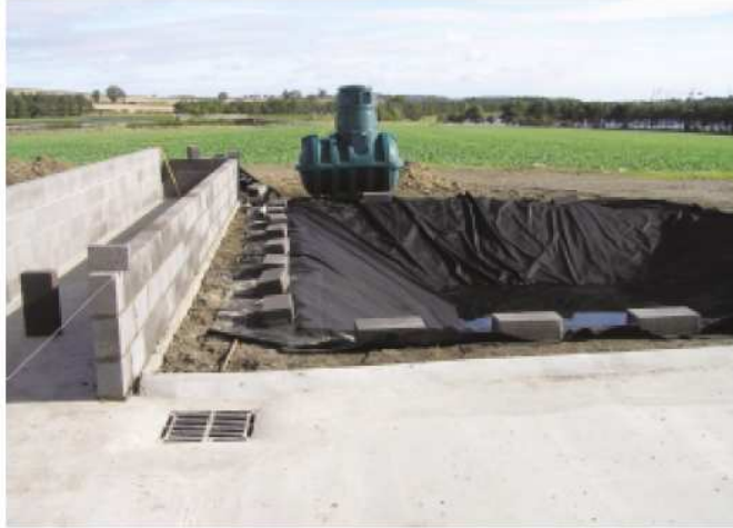
Plate 2 Indirect biobed system under construction. Bunded handling area in foreground, with a boom wash out section all draining to single collector. Background lined hole waiting to be filled with biomix and secure intercept tank awaiting installation.
