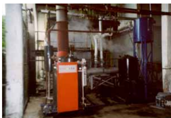
Figure 28 Pilot size hot press (top) and boiler to heat the press (bottom).
