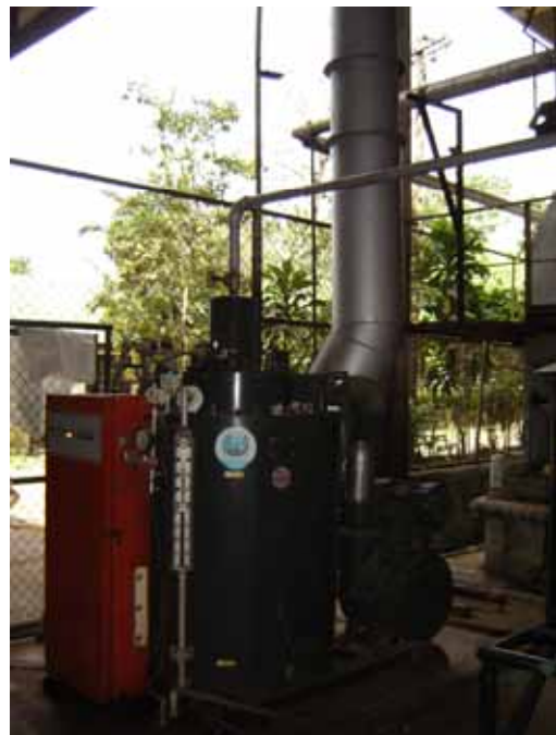
Figure 42 The steam generator
