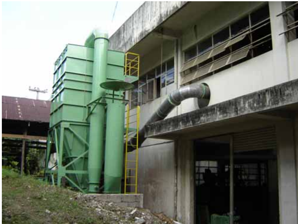
Figure 44 The air cleaning system
