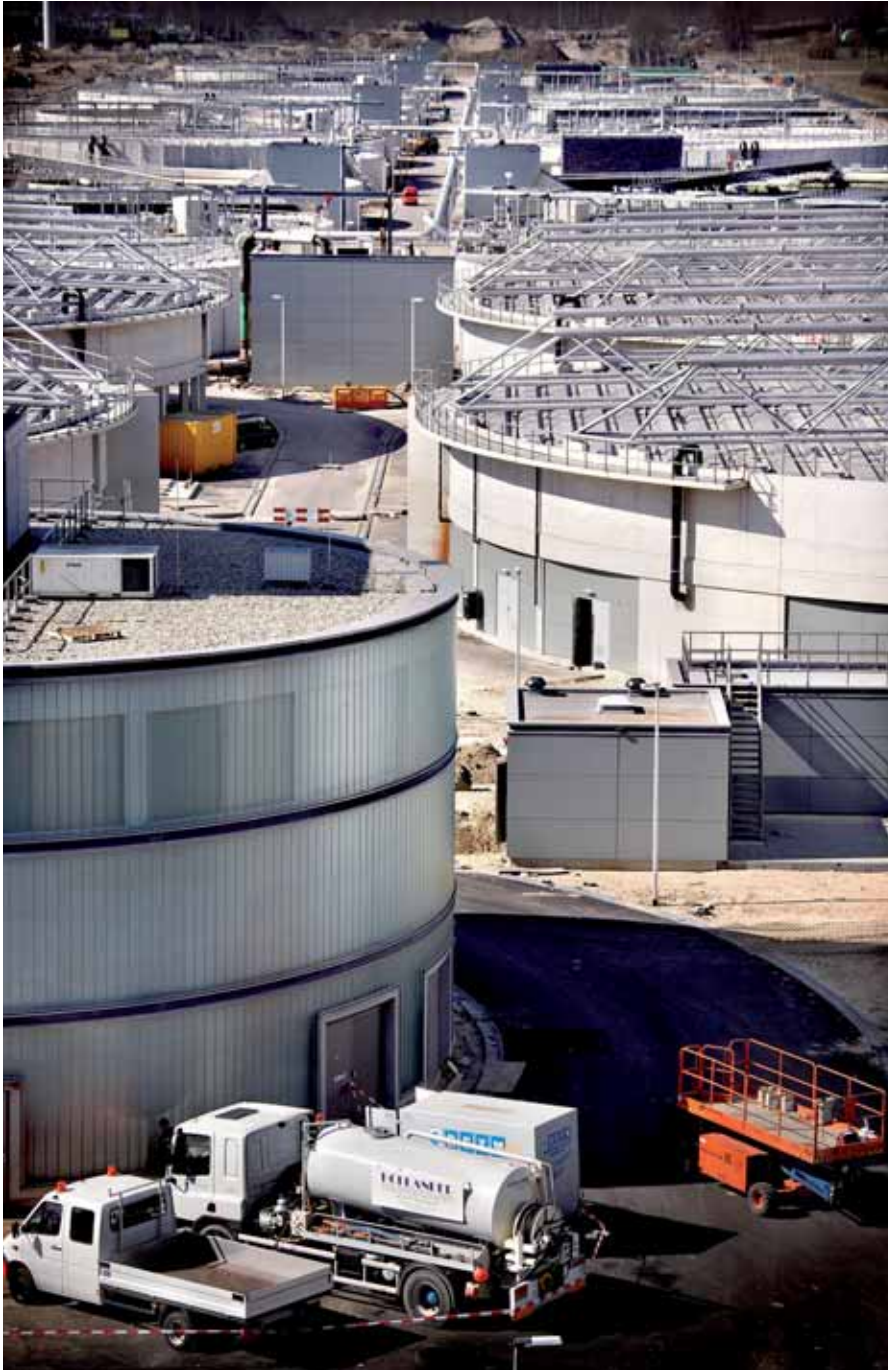
De rioolwaterzuivering in Amsterdam-West
