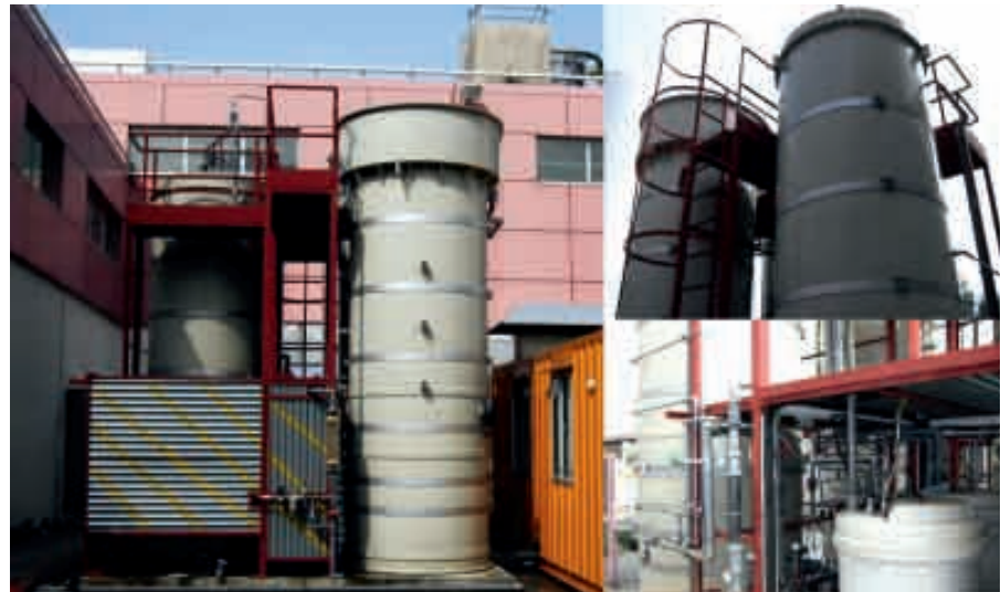
SANI-pilotinstallatie in Hong Kong.
