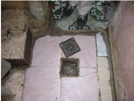
1. A not functioning infiltration tank
