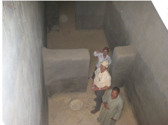
Septic tank (not well designed) to receive waste water of New Sheikh Masoud.
