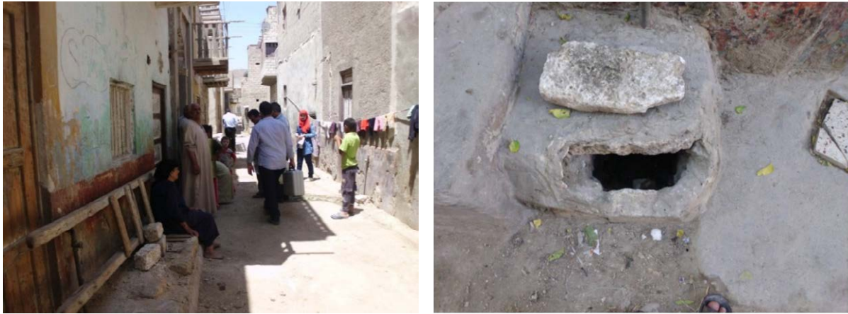
Photo 8 Left: Team identifying the sewage disposal system from bathrooms, toilets (solid waste and black water), kitchen, taps and other grey water (they have observed separation at large scale) Right: Pits for collection of solid waste and black water (discharged by cars once per year).
