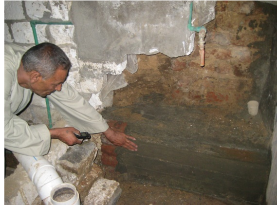
Wetting of the wall in the basement by waste water
