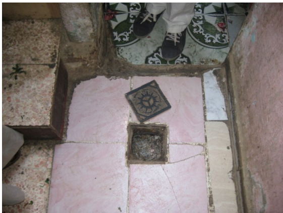
Non-functioning infiltration tank caused by high water table
