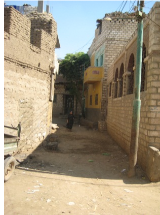
2. Wet walls caused by the high groundwater level.
