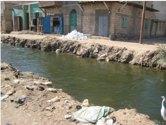
3. High water table in irrigation channel
