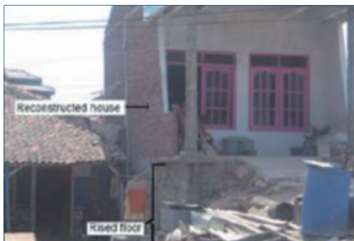
Figure 8 House and raised floor reconstruction (Marfai and King 2007b). The adjustments can be made by elevating the buildings on piles
