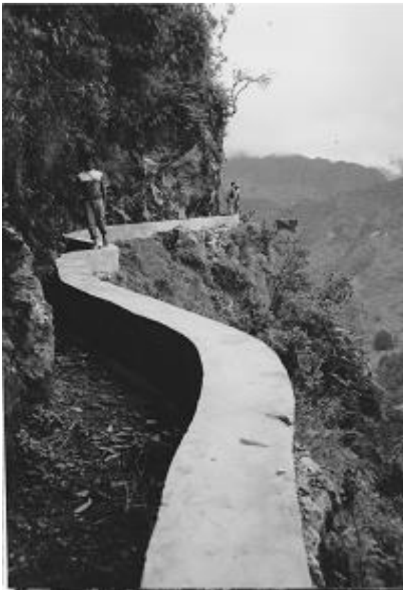
A newly constructed canal in the Mechi project (± 1990). Obtained from private collection
