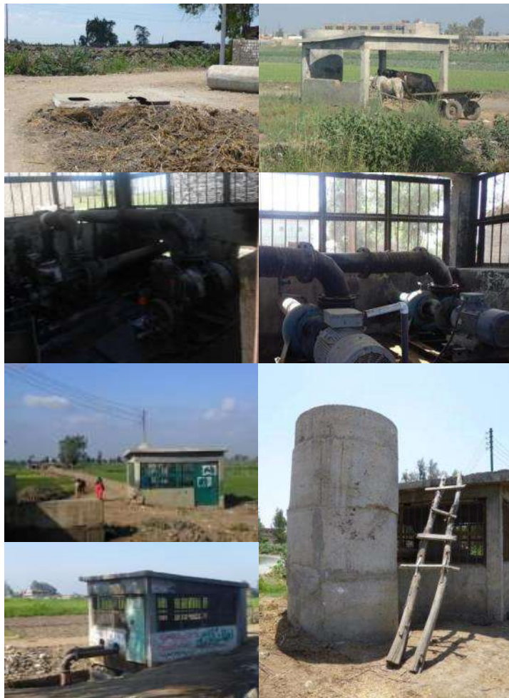
Figure 11 - Variety of IIP pumping stations along Abo Moustafa. They differ in operational status, engine type, power source and tower
