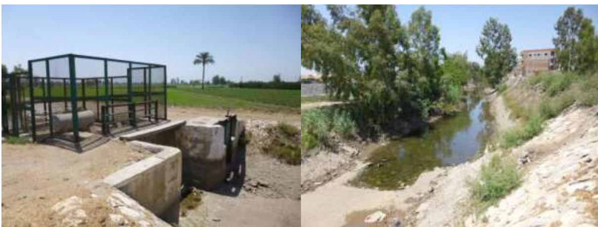
Figure 8 - AVIS gate in Abo Moustafa canal blocking water at low levels (6/6/2013)
