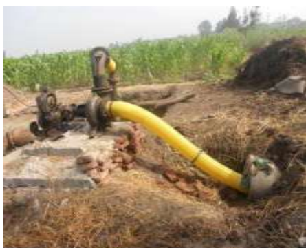
Figure 14 - An IIP diesel pump attached to the mesqa to pump drain water into the system (24/6/2013)
