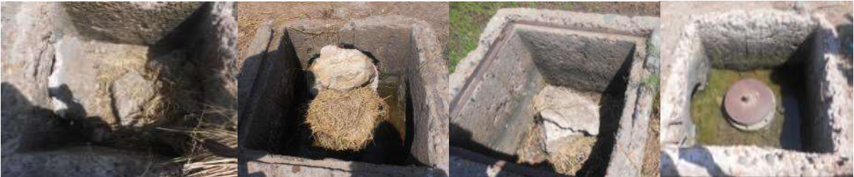
Figure 25 - Valves in PS33, varying from absent to broken to intact
