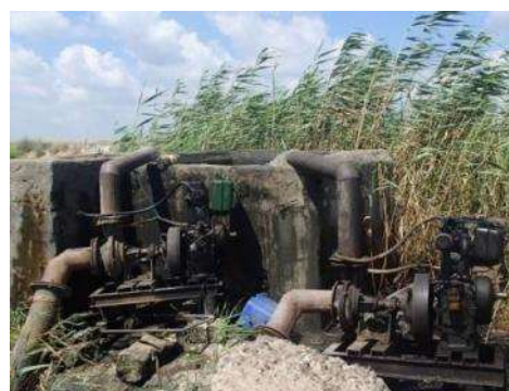
Figure 13 – Two newly bought diesel pumps attached to drain number 7 pumping water into the piped mesqa (16/6/2013)
