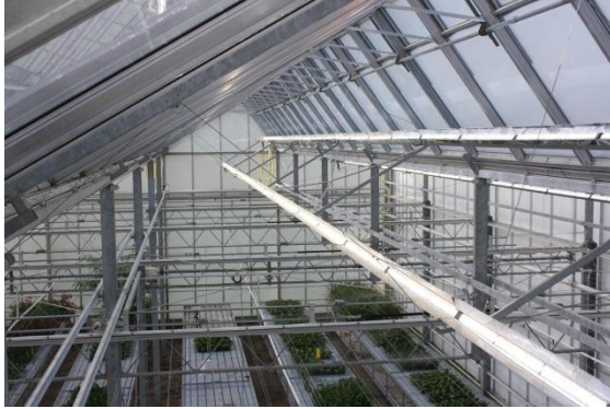
Fig. 1 PV collectors mounted in the roof of the greenhouse
