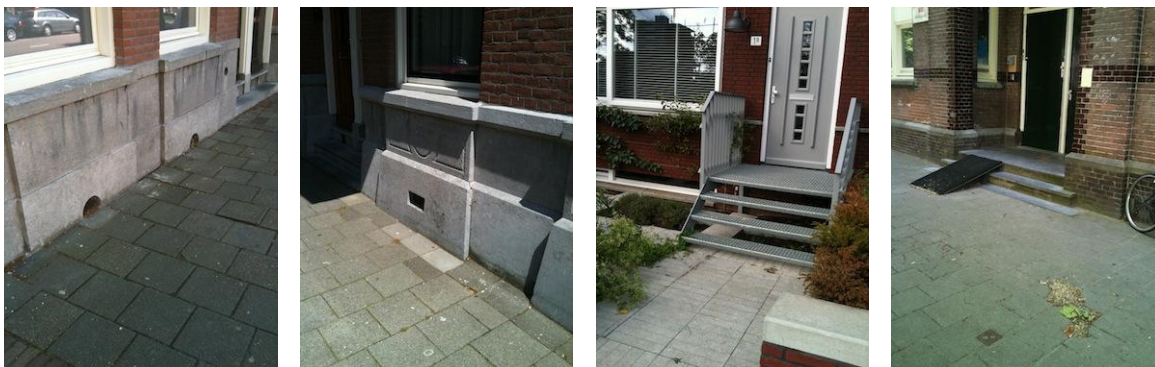
Photo 2.1 Height of air vents and door steps making properties susceptible for material damage
